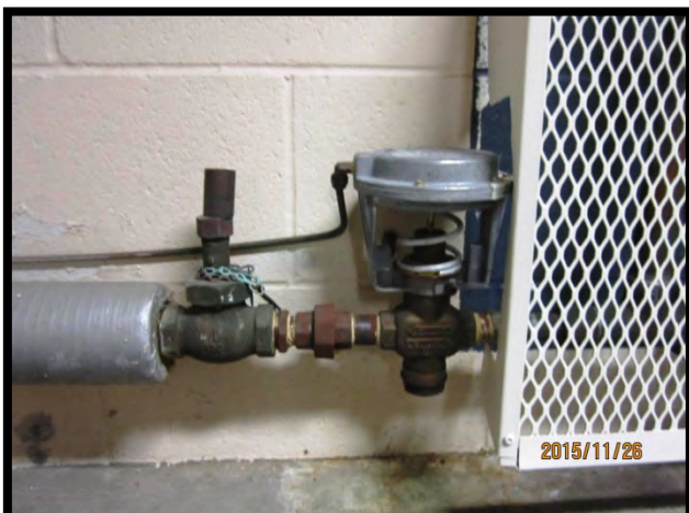
Zone control valves and pressure relief
