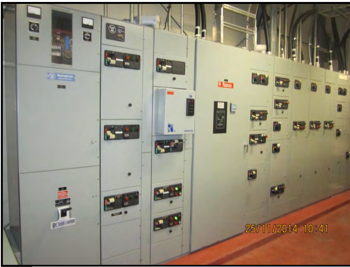
Motor Control Centre
