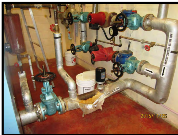
Hot water supply piping & pumps
