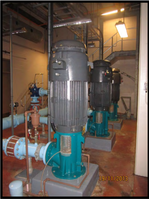
200 hp Distribution Pumps
