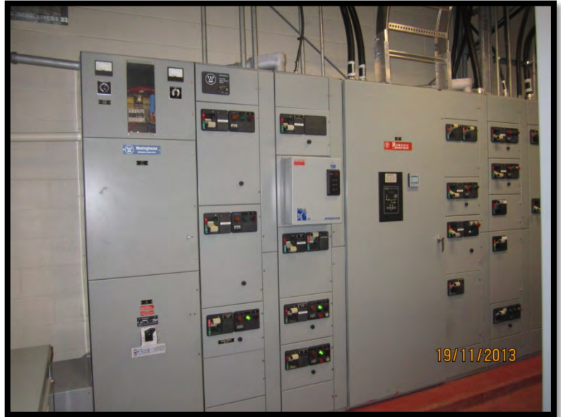
Motor Control Centre (MCC)
