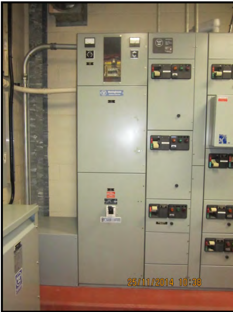
Main Incoming Breaker
