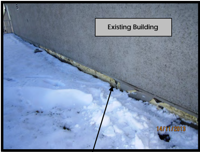
Cement Board Damaged
