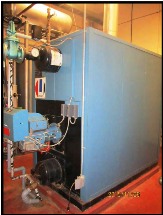
Existing 2,000,000 BTU boiler
